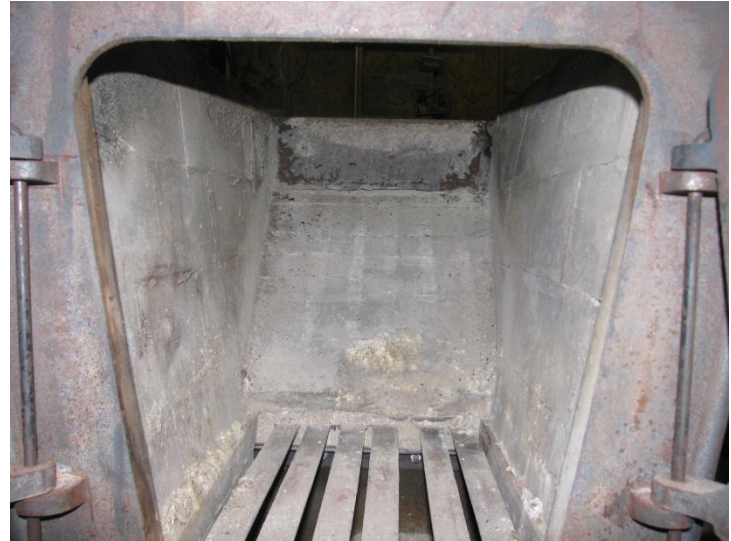
Picture of a bricked arch. High temperature cement is used lay bricks one against the other and to seal properly avoiding the heat to get through to the outside.
